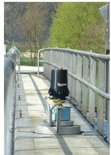
Slip ring assembly in circular scraper (sewage treatment plant)
