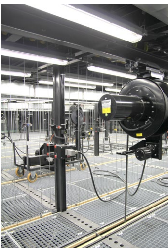
Slip ring assembly in theater (stage floor)
