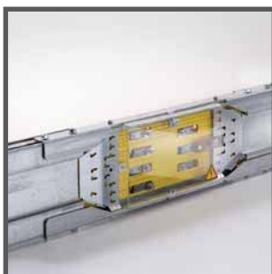
Additional power feed
